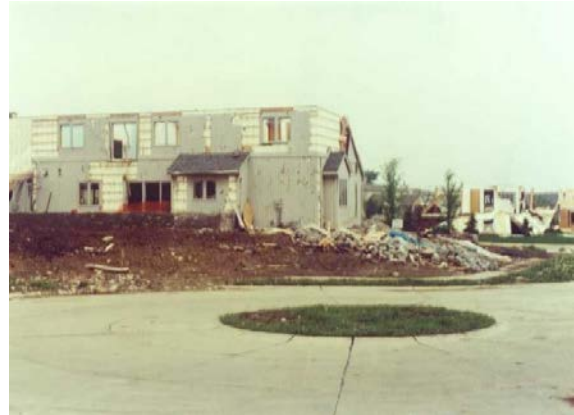
Figure 2: An ICF home survives a direct tornado strike with windows, siding, and roof destroyed.
